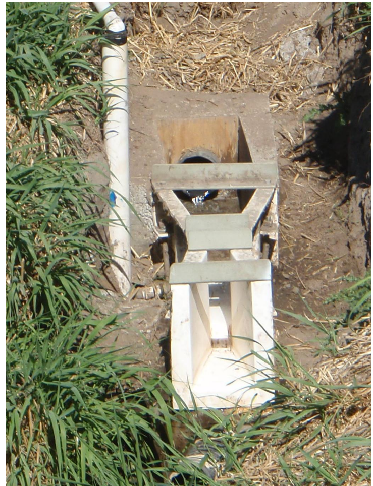
Drain Tile at CAF
